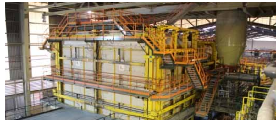
New furnace installed at Crisnova Vidrio.
